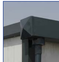
Rear Water Gutter System
